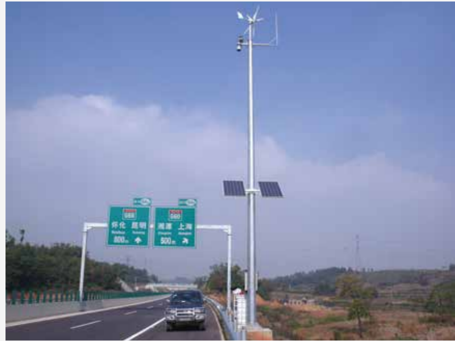
wind solar hybrid off-grid monitoring system for highway – Shaoyong Highway Guangzhou 2009
