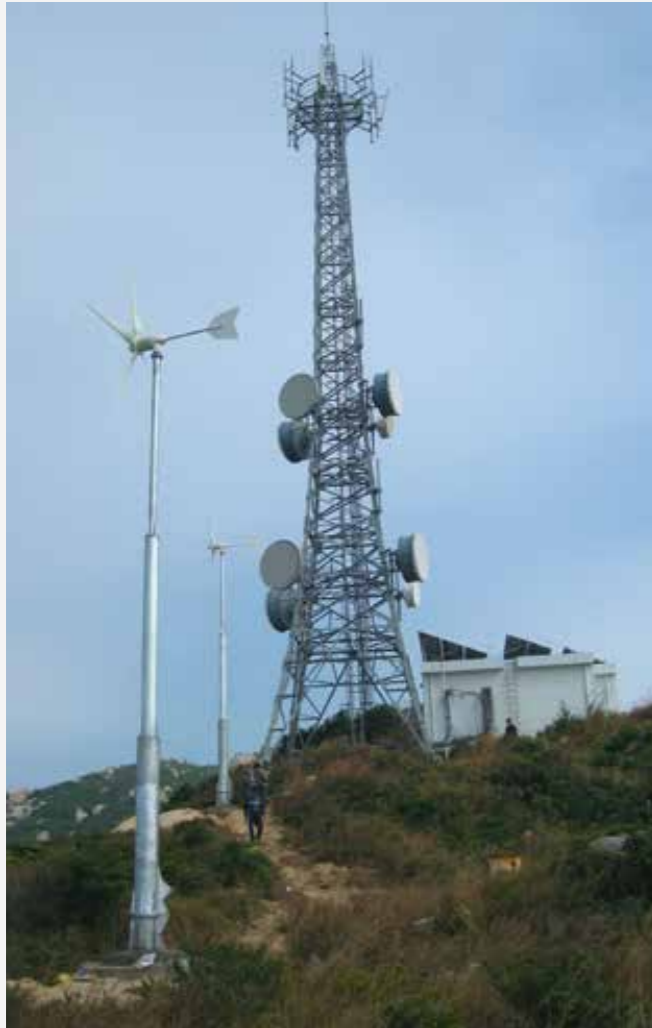
10KW wind solar hybrid off-grid power system for telecom tower – Baili Island, Zhuhai 2011
