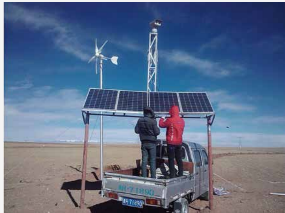
Wind solar hybrid off-grid monitoring system for oil field – Qinghai 2011
