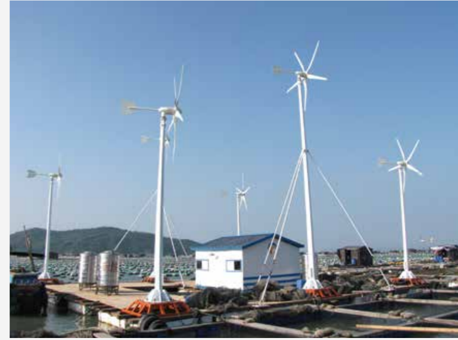
18KW wind powered stand-alone sea water desalination system - Bureau of Fishery, Fujian 2008
