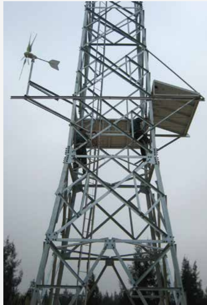
3KW wind solar hybrid off-grid power system installed on existing telecom tower as a backup power system – Hainan China 2012
