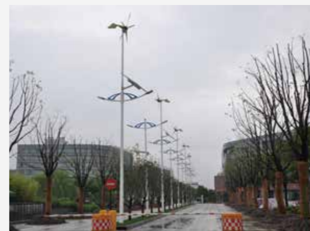
Pegasus 1 power 4 system 40 LED street light – Unionpay headquarter, Shanghai 2012
