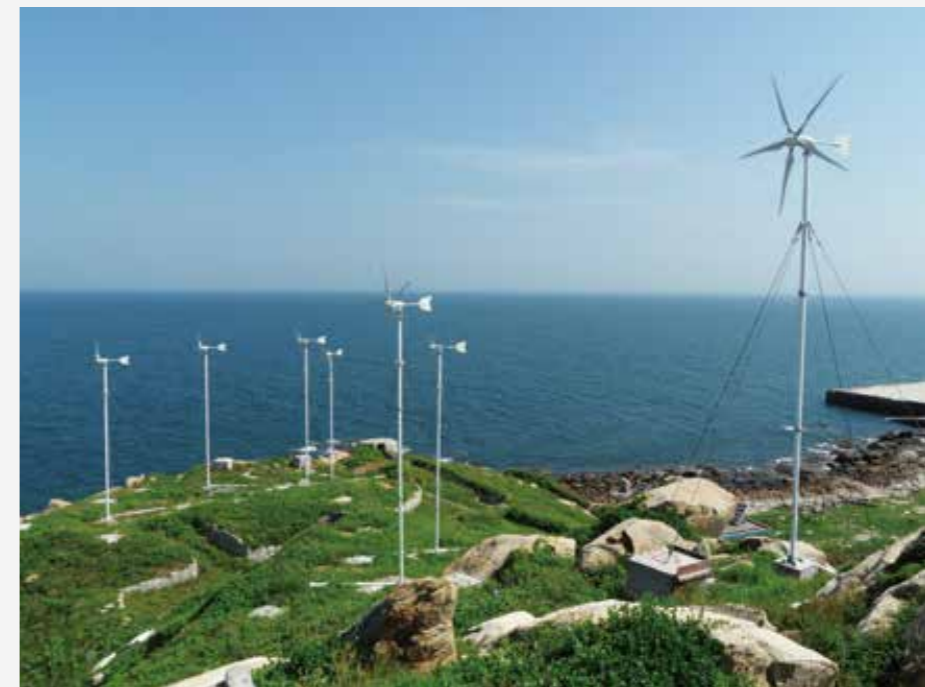
21KW wind powered stand-alone sea water desalination system – Nanpeng island, Shantou 2010
