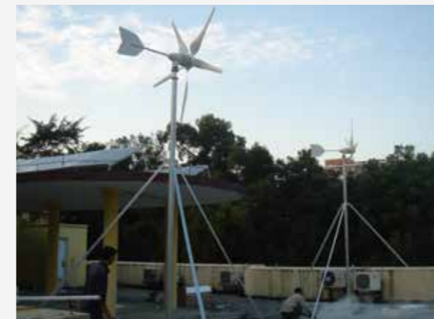
4KW wind solar hybrid off-grid power system for small business enterprise rooftop – South Korea 2010
