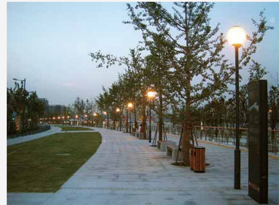
Total 33KW wind power array off-grid power system for eco-park lighting – 11pcs of DM-3000 wind turbine created off-grid system to power all lights of Binjiang Eco-green park, system is designed and constructed by DIMON– Shanghai 2010
