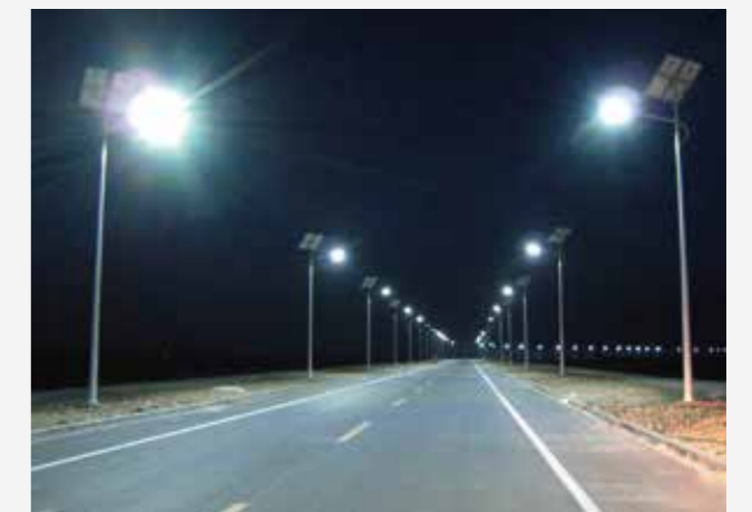
90W LED solar street light project – Denizli Turkey 2012
