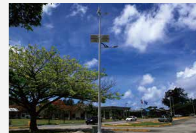
60W LED wind solar hybrid street light – Saipan Island, CNMI - 2009
